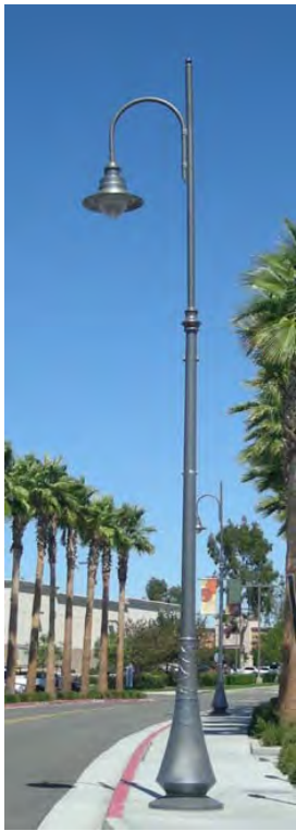
Commercial Parking Lot Lighting
