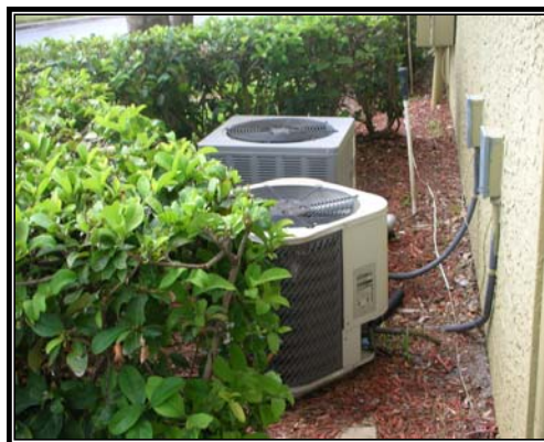
Landscaping is one alternative for screening ground-mounted equipment from public view.
