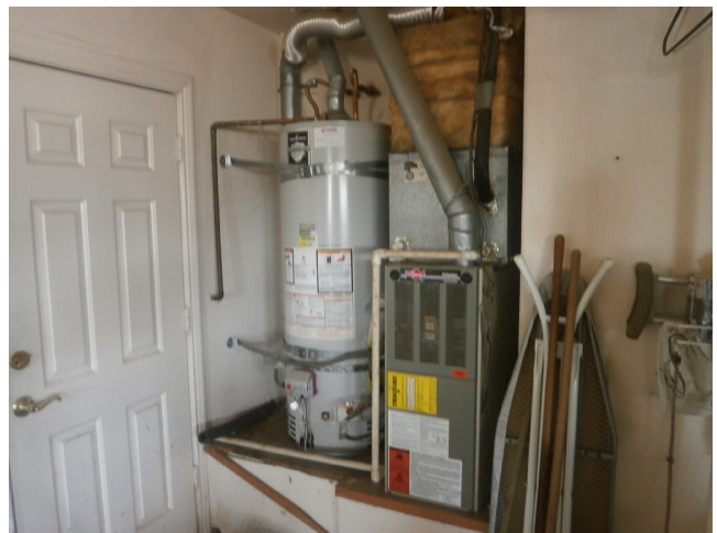
Water heater and furnace
