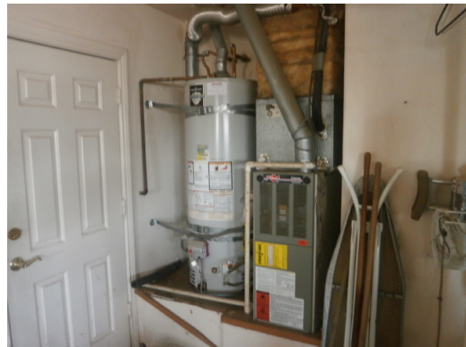
PHOTO #16 WATER HEATER AND FURNACE
