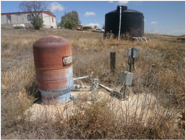
Water well and water storage tanks
