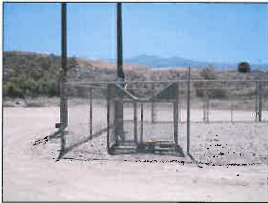
PHOTOGRAPH 8: View of East Valley Water District well.
