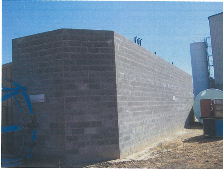
Proposed block wall encasing all tanks
