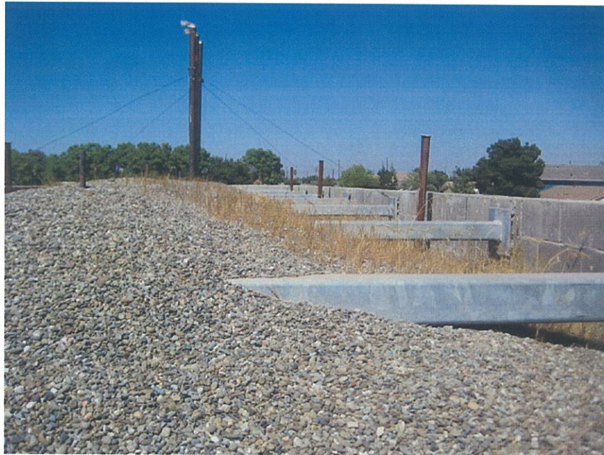
Pea gravel that buries tanks and structural metal support beams.
