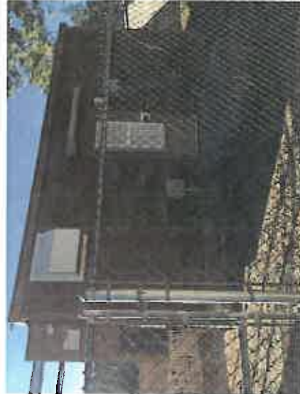
Close-up view of equipment shelter from the east side within Idyllwild Fire Station fence
