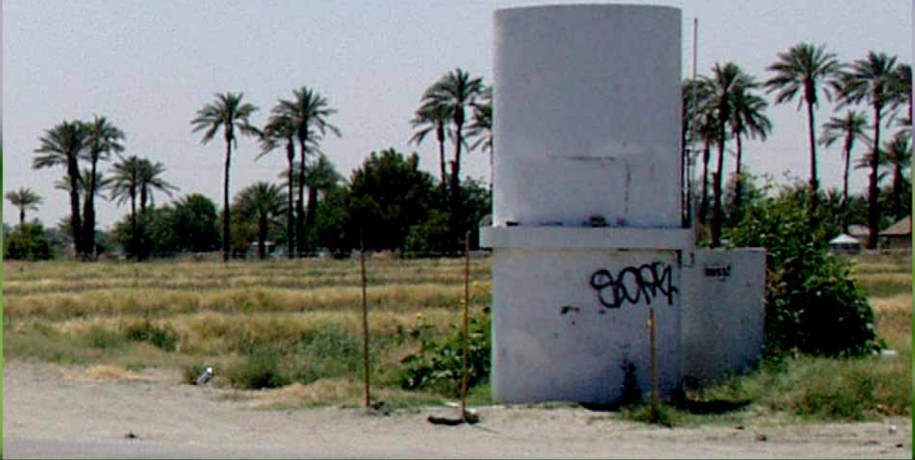
Pressure Regulator Pipes
