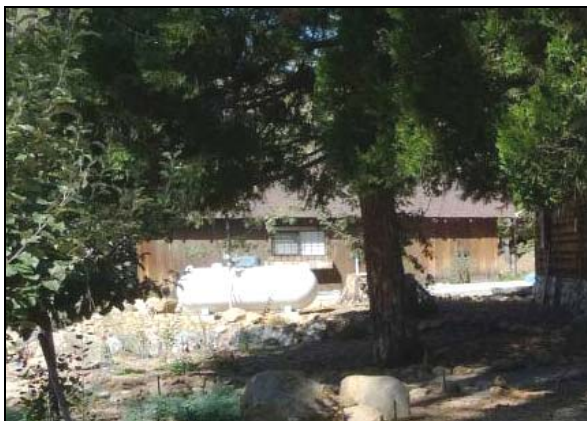
Figure 40: Exposed propane tank
