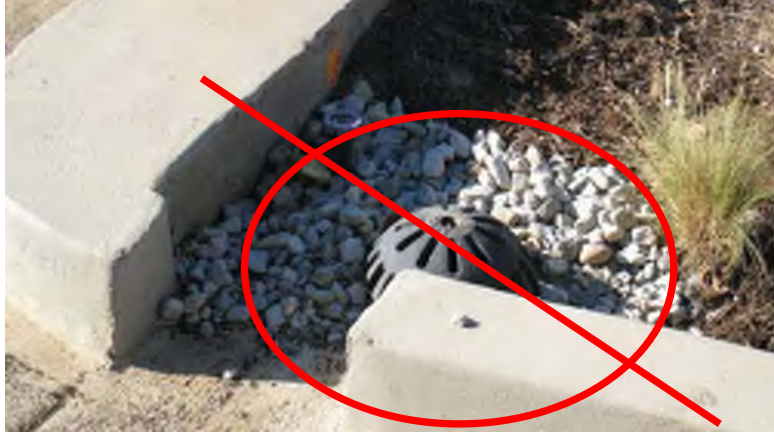
Figure 6: Incorrect Placement of an Overflow Inlet.
