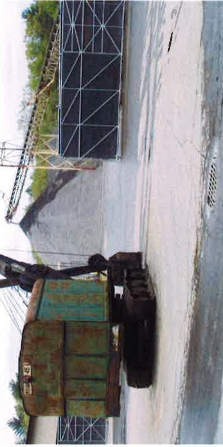
Storm drain adjacent to access road to plant; drain is not protected and not being serviced.
