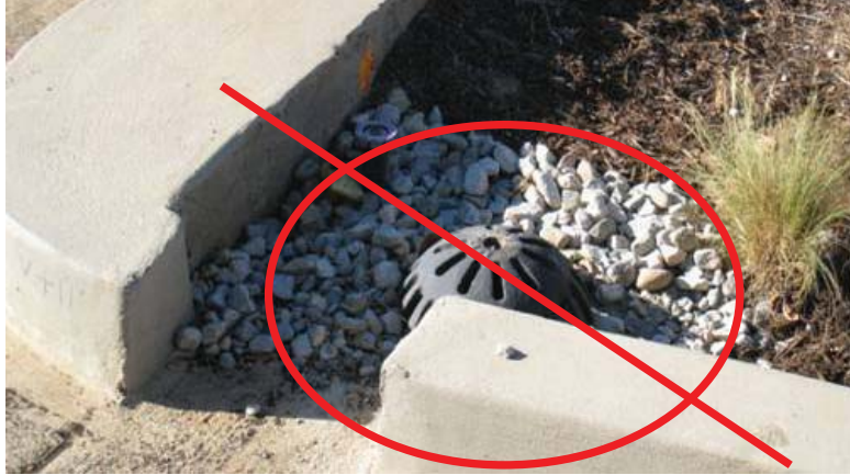
Figure 6: Incorrect Placement of an Overflow Inlet.
