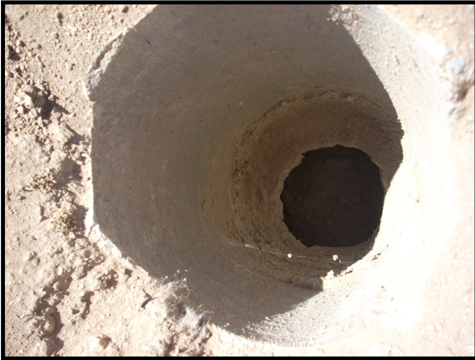
Photo P-9 – View down one of several concrete pipes extending into the subsurface.
