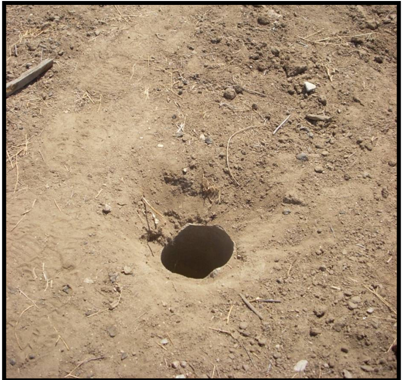
Photo P-8 – One of several concrete pipes extending into the subsurface. Likely associated with a former irrigation system.
