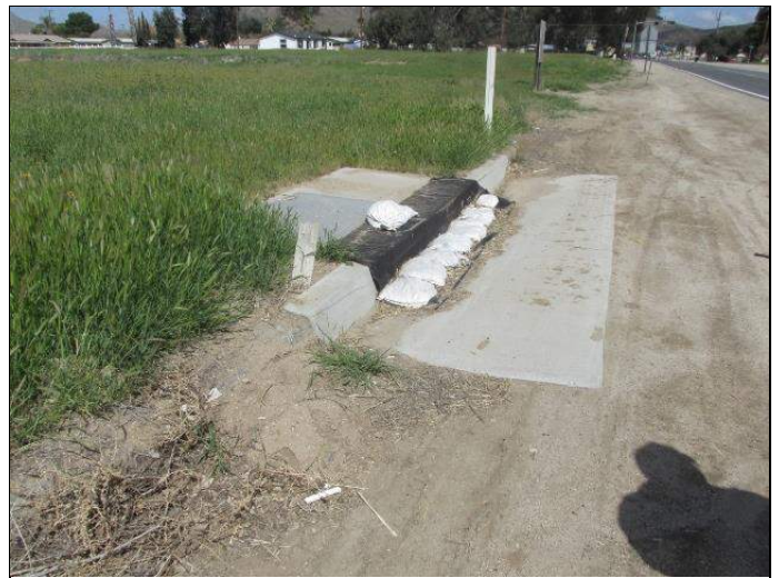
4. View of a stormwater drain: not in use.
