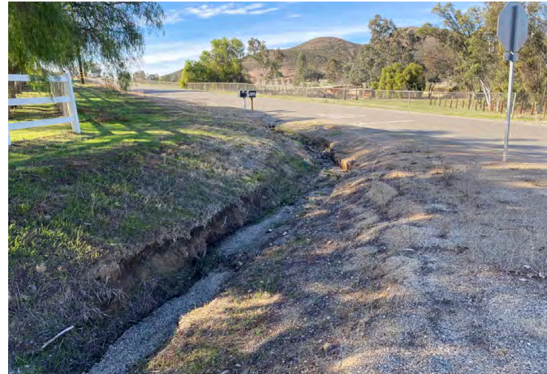
Photograph 20: 02/03/21. Roadside ephemeral Drainage I located in offsite survey area.
