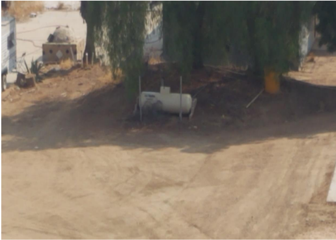
An aboveground storage tank for propane.
