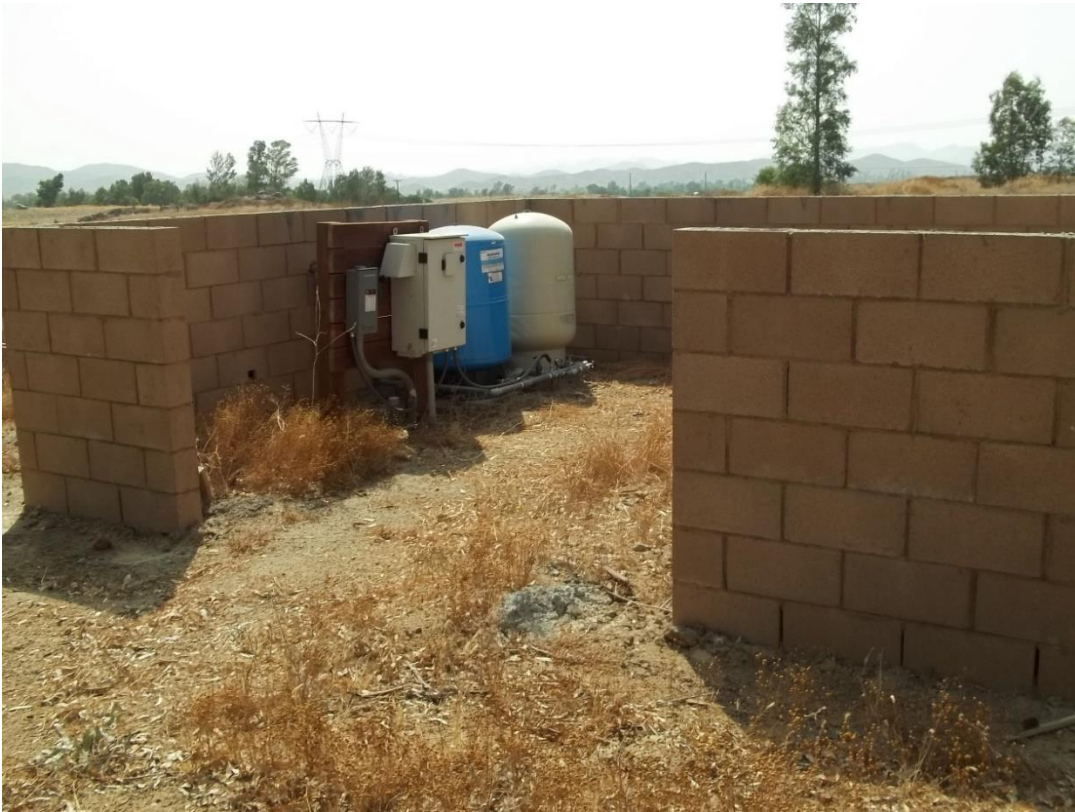
Water softener drums located on the southern portion subject site.
