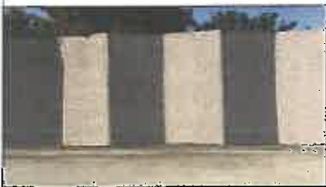
EXISTING ZIG-ZAG BLOCK WALL LOCATED ALONG A PORTION OF THE SOUTH PROPERTY LINE ZIG-ZAG WALL TO REMAIN AND REPAINTED
