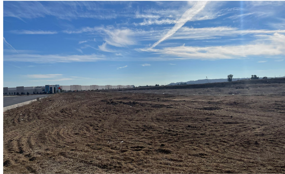
Site Photo 14-2: From northeast corner of the project site, along Commerce Center Dr, facing southwest.
