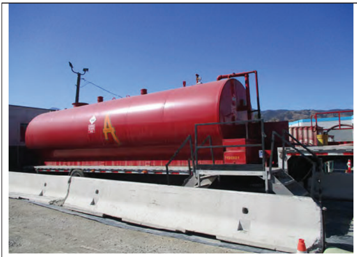
15. View of a diesel AST at Ames Construction.
