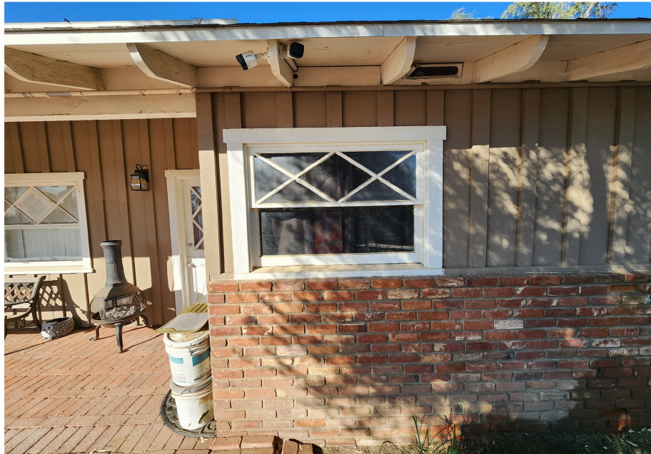
Plate 4.3–12: View of a window on the east façade of the 23330 Walnut Street residence, facing west.
