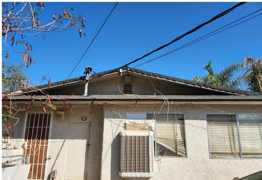
Plate 4.3-36: South façade of the 20111 Patterson Avenue residence showing the vent in the gable end, facing north.
