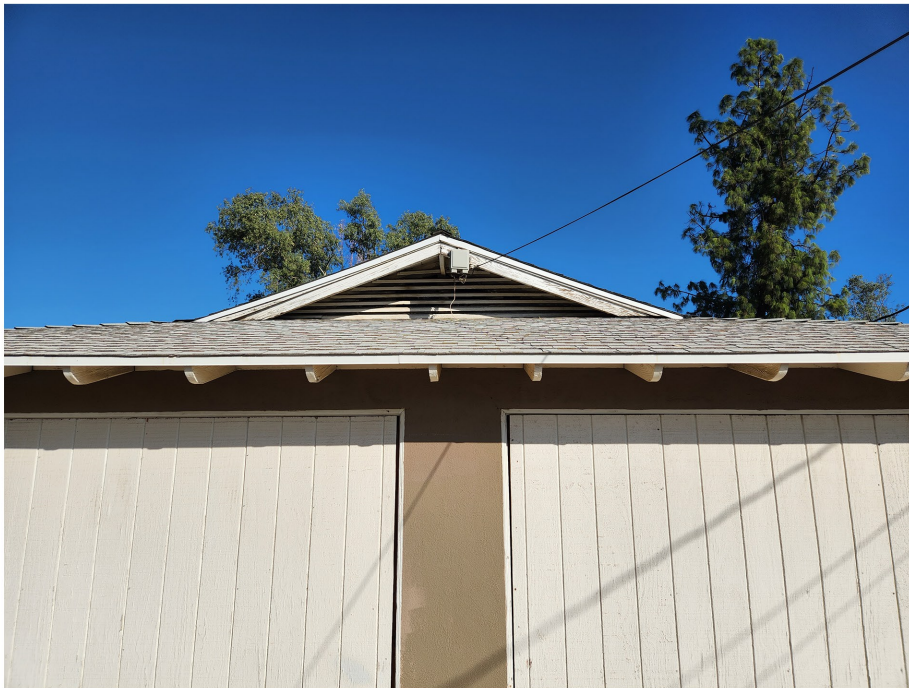
Plate 4.3–18: South façade of the 23330 Walnut Street residence showing the vent in the gable end, facing north.
