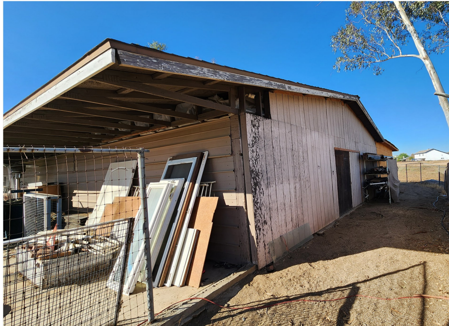
Plate 4.3-21: Southeast corner of the 1977 to 1990 garage/barn on the 23330 Walnut Street property, facing northwest.
