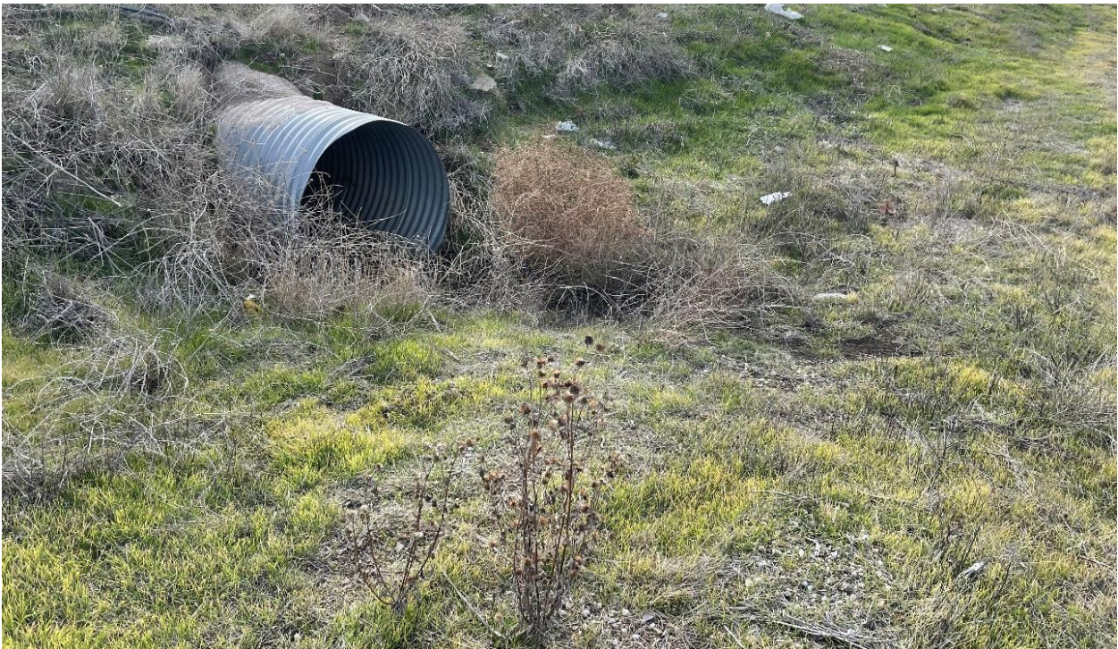
Photograph 6. Culvert under Highway 79 (Winchester Road) northeast of the intersection with Pourroy Road/Abelia Street.
