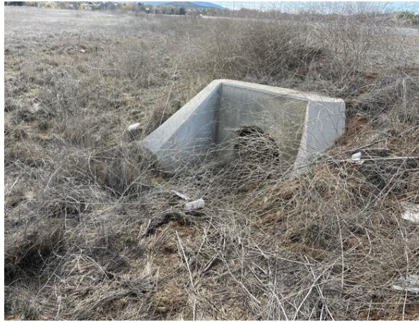
Photograph 2. Storm drainage adjacent to SR 79
