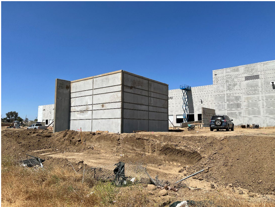
Photo 14 – Building under construction to the west of the western portion of the Property.
