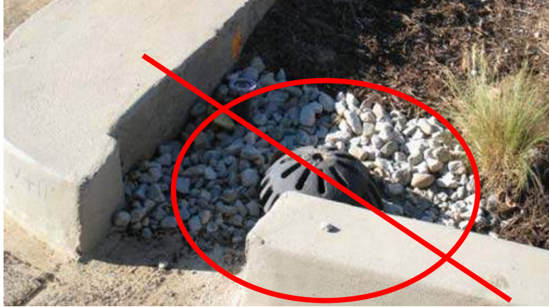
Figure 6: Incorrect Placement of an Overflow Inlet.
