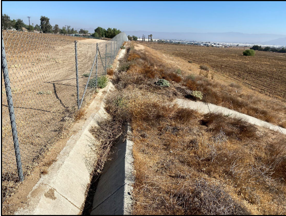
Plate 4.2-2: Overview of the concrete v-ditch system along the western boundary, facing north.
