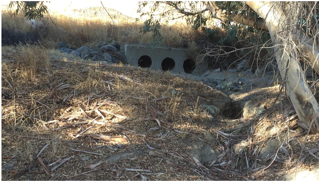
Plate 4.2–4: Overview of the culverts located within the man-made Cold Water Creek Channel, facing west.
