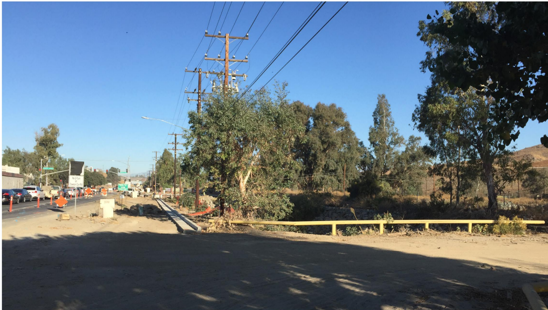
Plate 4.2-5: Road improvements currently being conducted on Temescal Canyon Road along the western boundary of the project, facing north.
