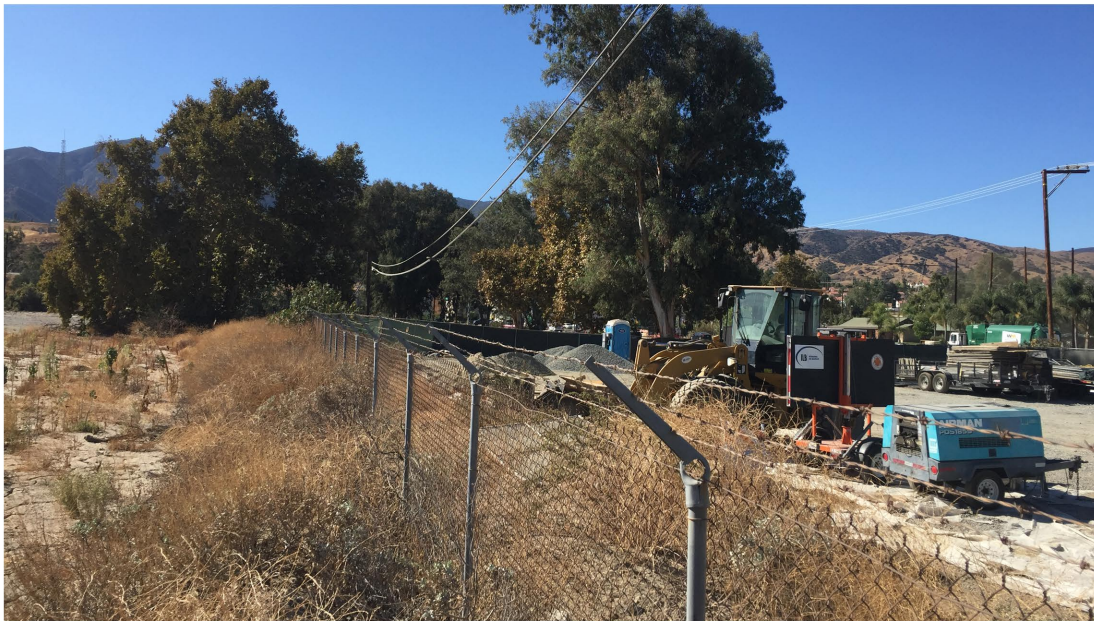
Plate 4.2-6: View of the northern portion of the project currently being utilized for the staging of equipment, facing northwest.
