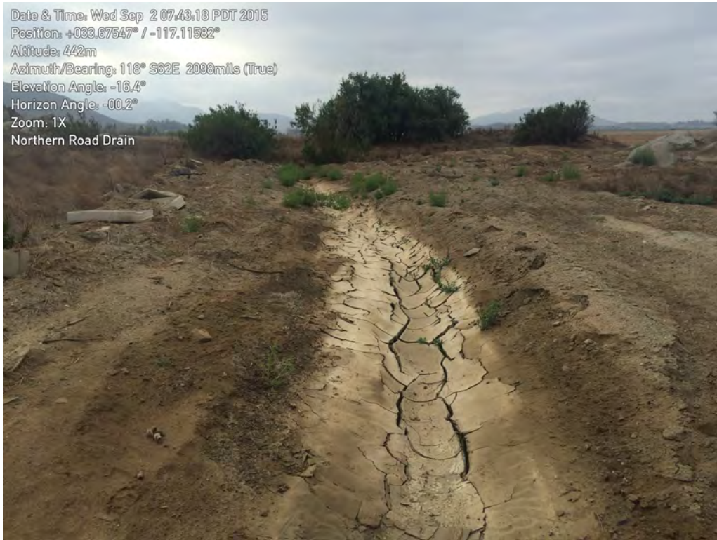
Photo 1. Connection of northern road drain to Leon Road with northern road drain impounded area visible in the background. Survey results were negative for fairy shrimp eggs.
