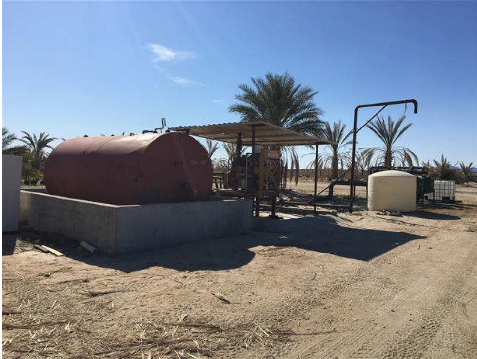
AREA F: Fuel AST with secondary containment, irrigation well, pumping, and filtration equipment.
