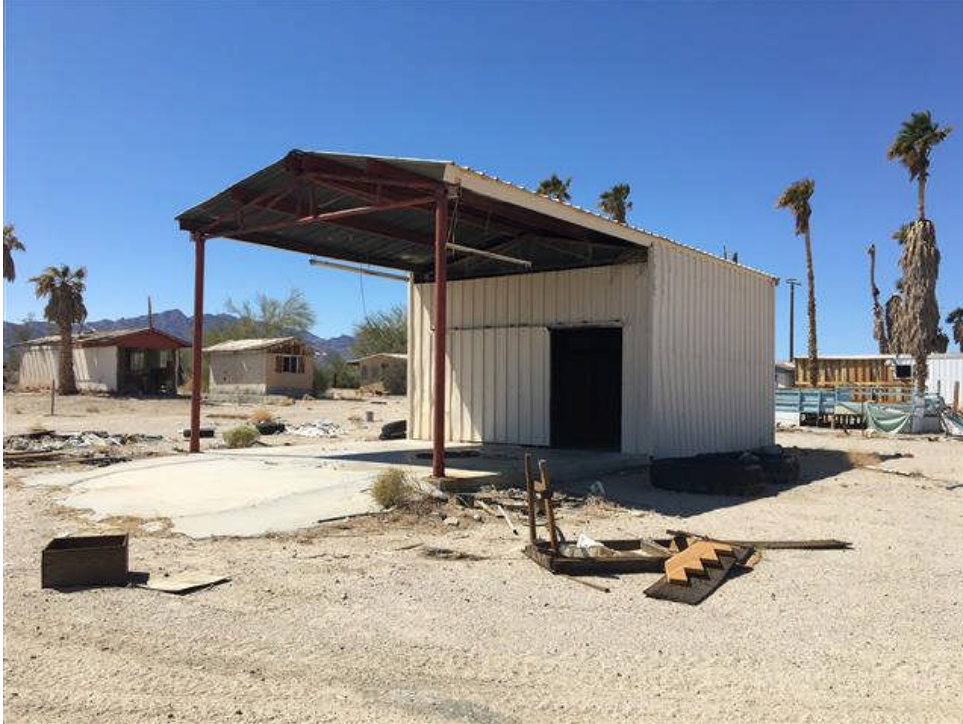
AREA B: Apparent shop building in the southwest portion of Area B. No staining or subsurface structures were noted.
