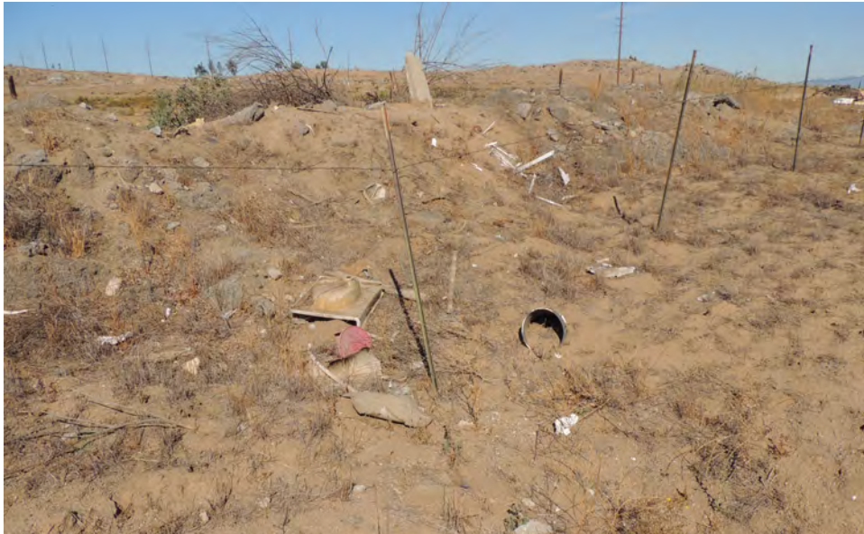
Berm located on the east side of Decker Road. This structure has completely isolated the swale from receiving upstream hydrology.
