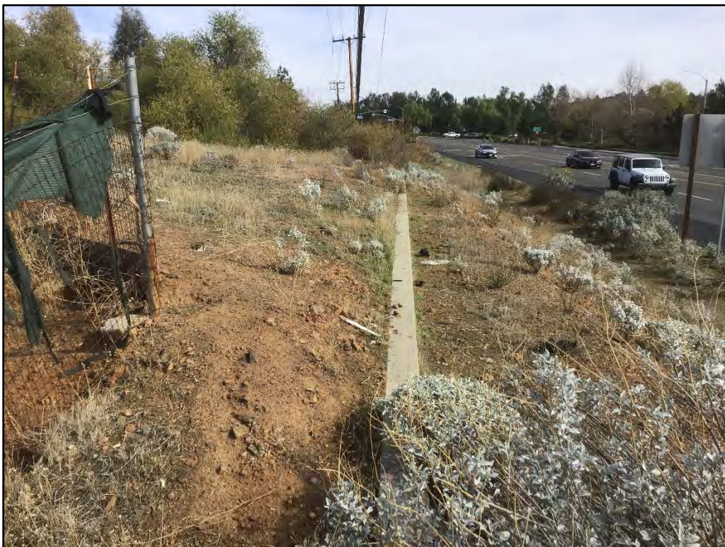
Figure 6. Overview of modern retaining wall/curb along southeast border of Project Area, facing northeast.
