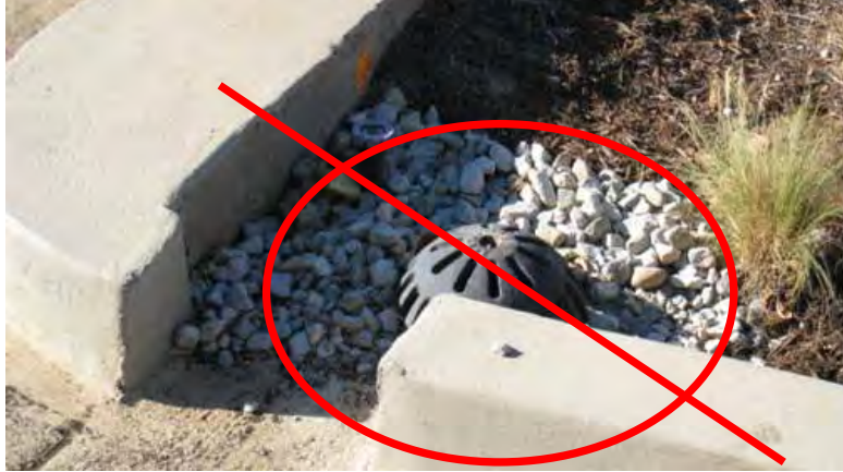
Figure 6: Incorrect Placement of an Overflow Inlet.
