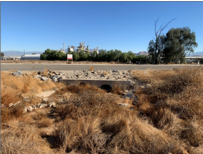
33. Stormwater culvert drain on the northeast boundary of Parcel A, view facing east.
