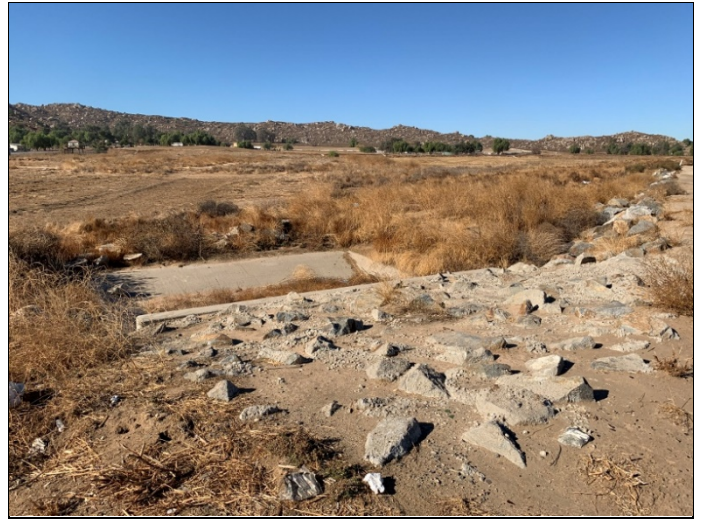
32. Stormwater culvert drain on the northeast boundary of Parcel A, view facing west.
