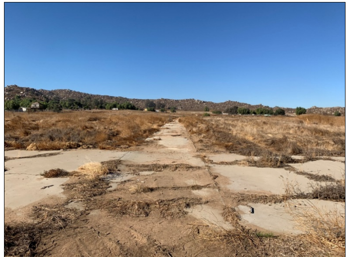
34. Foundations north of the abandoned building on the northwest portion of Parcel A, view facing west.
