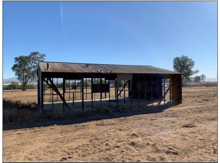
20. Abandoned building on the northwestern portion of the subject property, view facing southeast.
