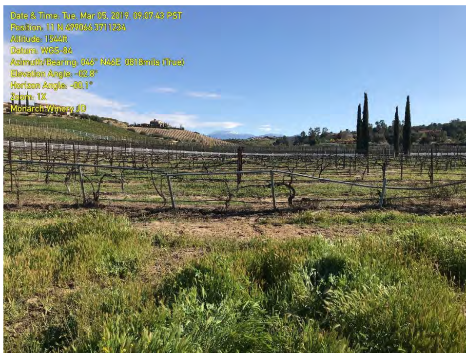
PHOTOGRAPH 11: The Property fence-line was bent and damaged in the upstream end indicating that strong surface sheetflow with debris (i.e., some Russian thistle was present on east side of fence) encountered this area. The fence-line likely dissipates flows since evidence of concentrated flow downstream of the fence was absent.
