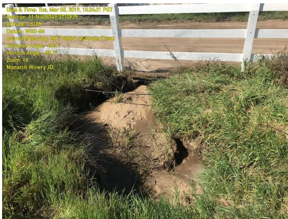
PHOTOGRAPH 2: Flow concentrating, then exiting the Site beneath a vinyl fence lined with wire.
