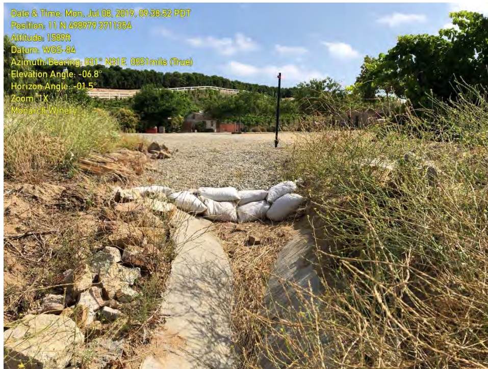
PHOTOGRAPH 17: A concrete V-channel and sandbags offsite above where the erosional gully originates.
