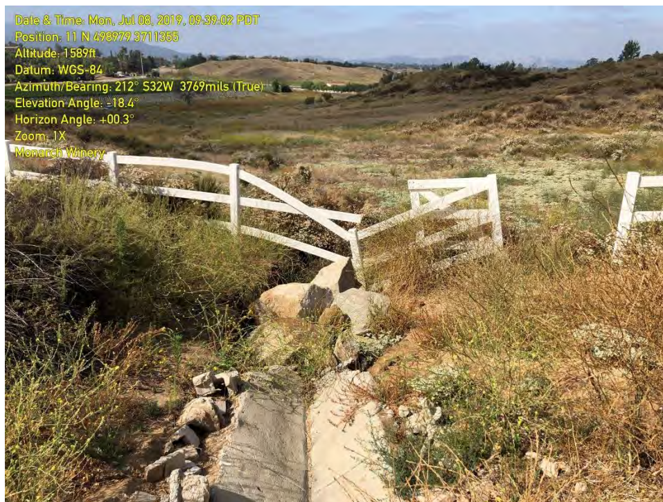
PHOTOGRAPH 18: A view of the same area looking downstream towards the Site. The boundary is at the fence.
