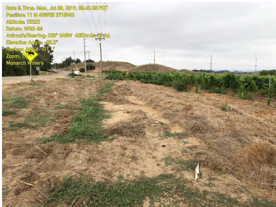
PHOTOGRAPH 6: No clear roadside drainage or Riverine feature was present downstream of the culvert conveyance area indicating flows dissipate to sheetflow.
