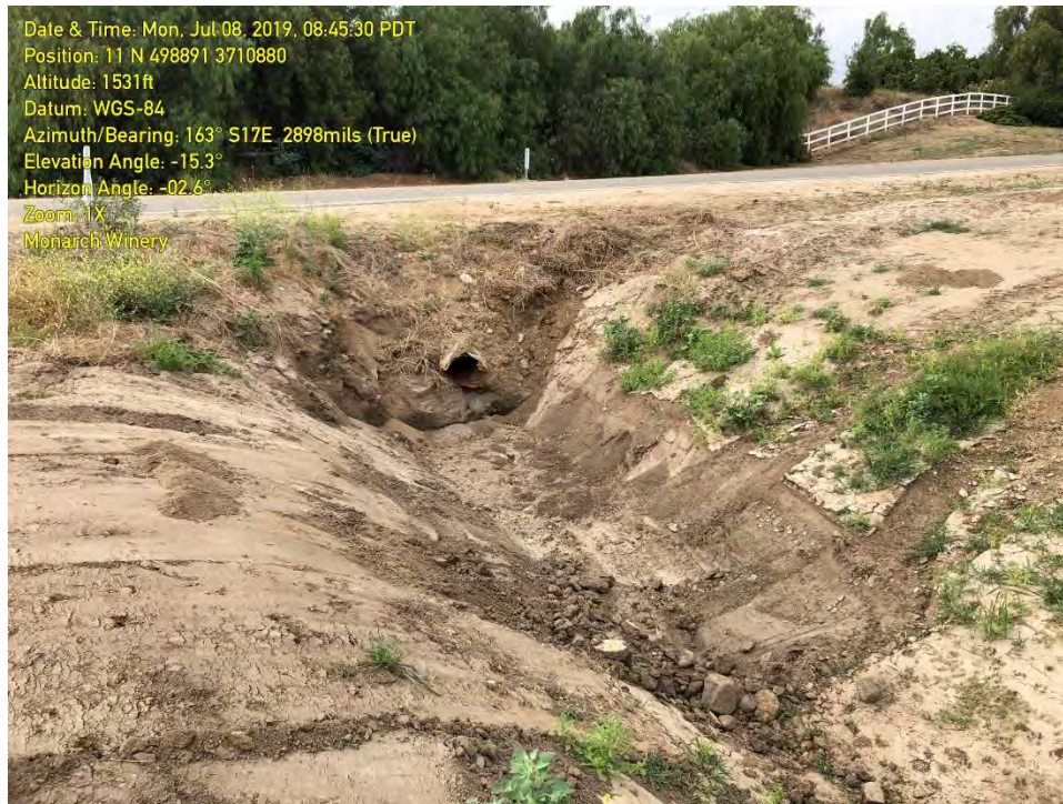
PHOTOGRAPH 7: A single 24-inch culvert conveys flows from the eastside of De Portola Road to this collection area.
