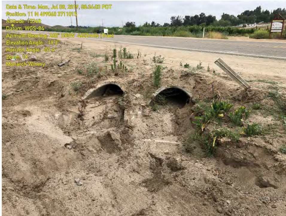
PHOTOGRAPH 3: Sediment has built-up within two 24-inch culverts where the roadside drainage enters.
