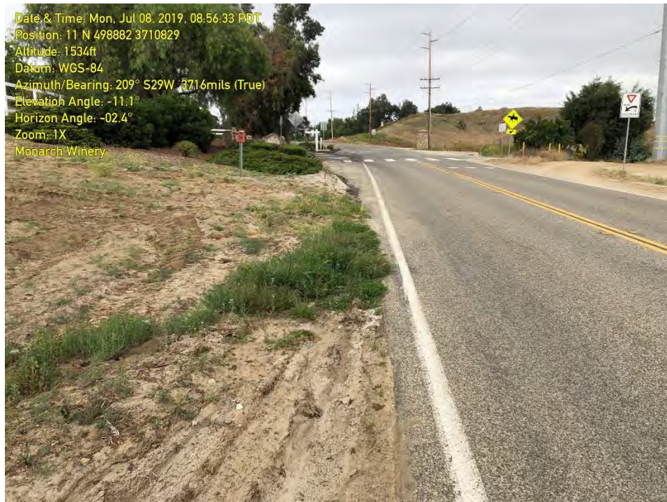
PHOTOGRAPH 10: The area where road runoff enters the human-created channel.
