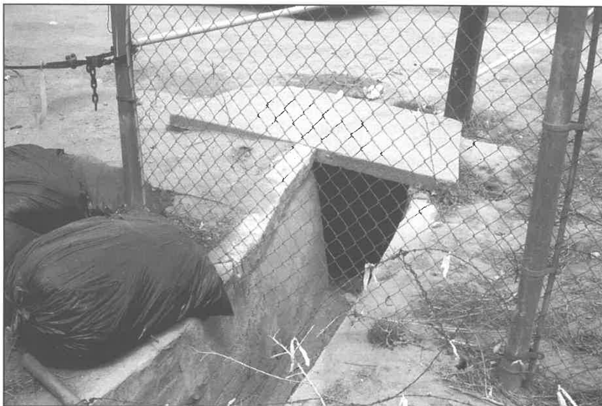
Image032.jpg: Site entrance to buried pipe in Center Street.
