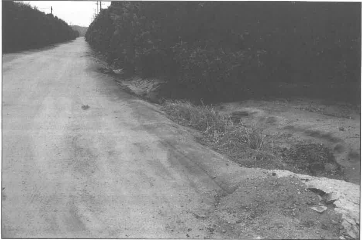
Image049.jpg: View of site at far western end near the intersection of Mount Vernon Avenue and Spring Street. View east.
