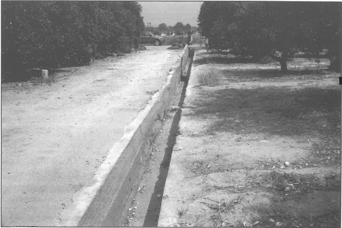
Image031.jpg: North view of site a few dozen feet south of Center Street. Most of the ditch is composed of rock and mortar with applied cement facing.
