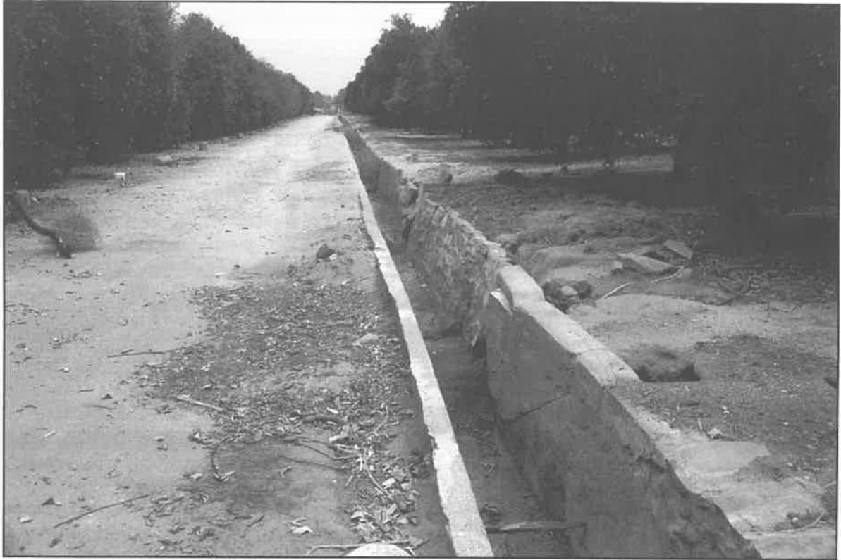
Image027.jpg: North view of site a few dozen feet of standpipe complex. Note collapsing sections that have been repaired with stone and mortar.
