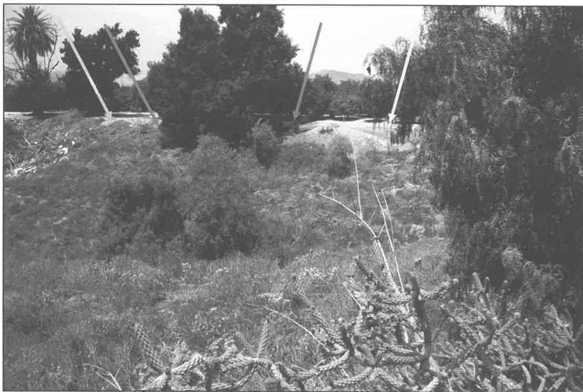
Image066.jpg: View of poured concrete portion of wall near south end (views are limited by vegetation). Collapsed area discussed in text indicated by the blue arrow. The intact area of concrete is found beneath an oak and the red arrows indicate the location. The green arrow indicates southernmost portion of the stacked cement block section of the wall.
