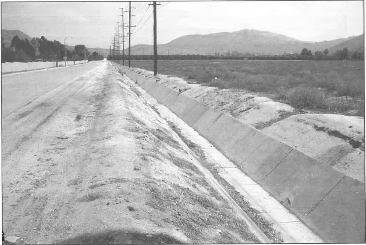
View of project area along Spring Street toward center body of proposed project. Modern concrete flume here replaced an older cobble flume.
