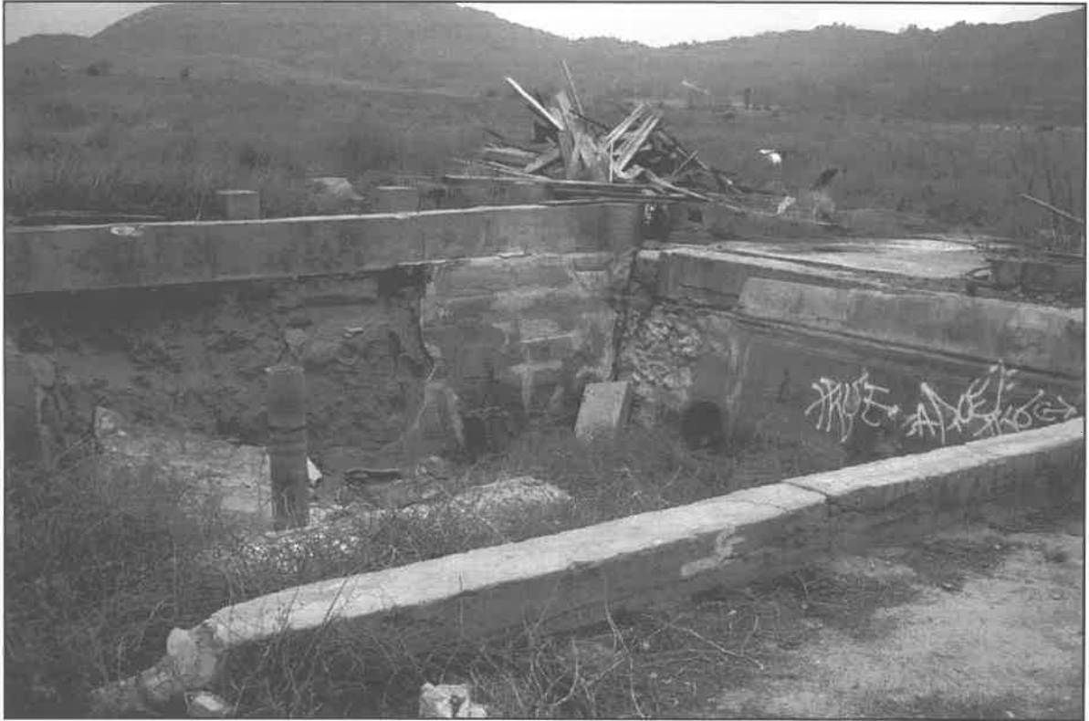
Image015.jpg: View of Feature 2 pump house reservoir and remaining wood framing. Reservoir is about 12 feet deep. Pumps were probably placed on the concrete slab to toe south (right). View to the southeast.
