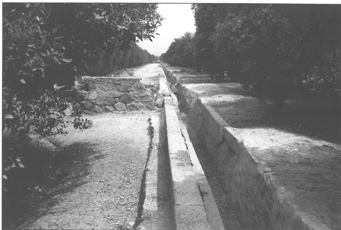
Image023.jpg: View of canal/retaining wall site near the center point to the north. Standpipe and brick reservoir to the left are not actually part of the site. These are associated with a gravity-fed irrigation delivery system and not the runoff collection system of CA-RIV-4198/H.
