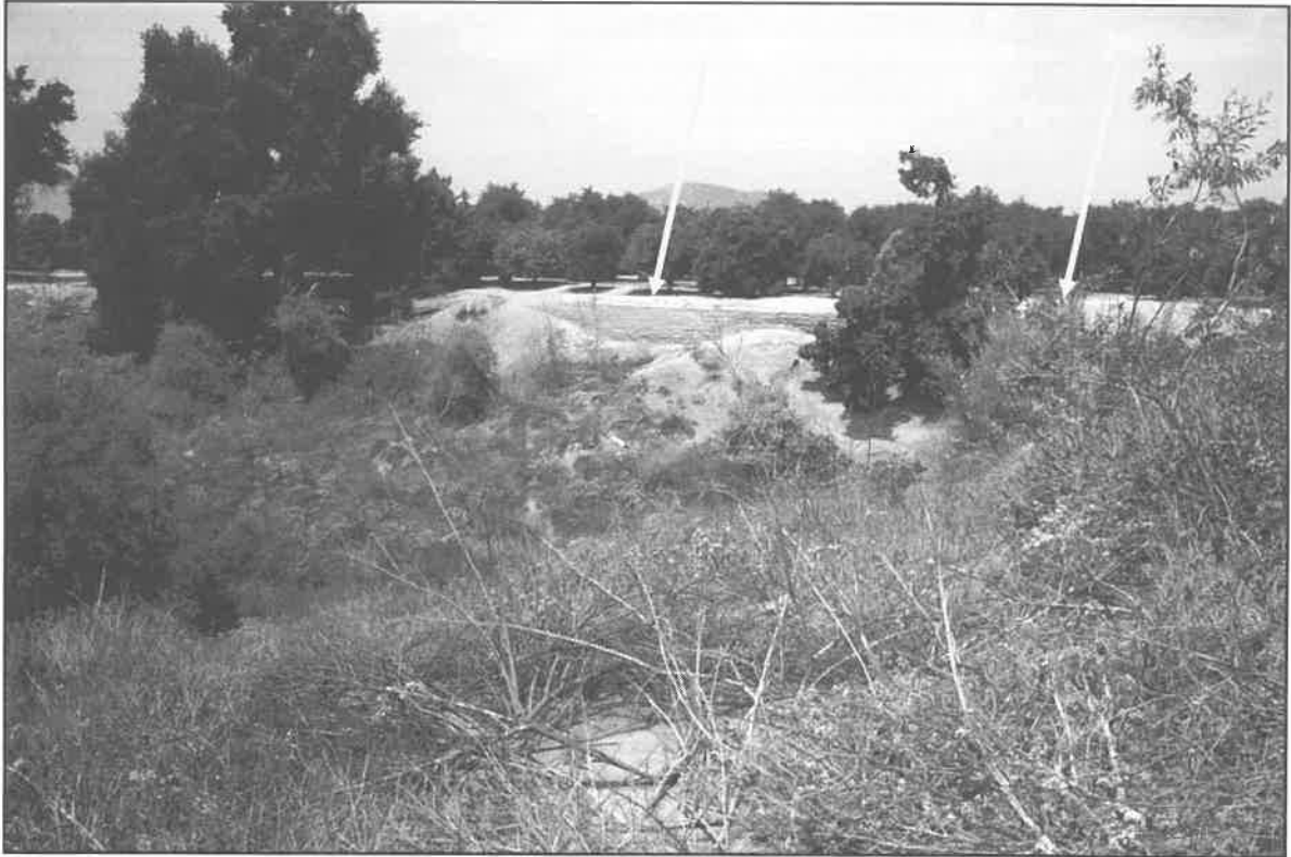
Image067.jpg: View of stacked cement block section of the retaining wall, with green arrows indicating location. That portion to the left (green arrow) can be seen in the following photograph. A small orchard seen in the archival photo below (possibly watered by outflows from SMO-4) was located on the flat land found at the base of this site.
