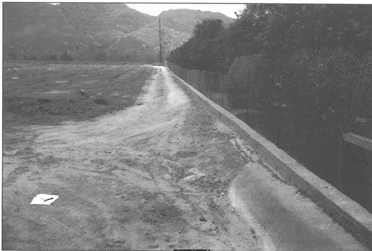
Image020.jpg: View of the site from the center point south along a possibly modern poured concrete retaining wall. Wall ends 100 feet north of Spring Street.
