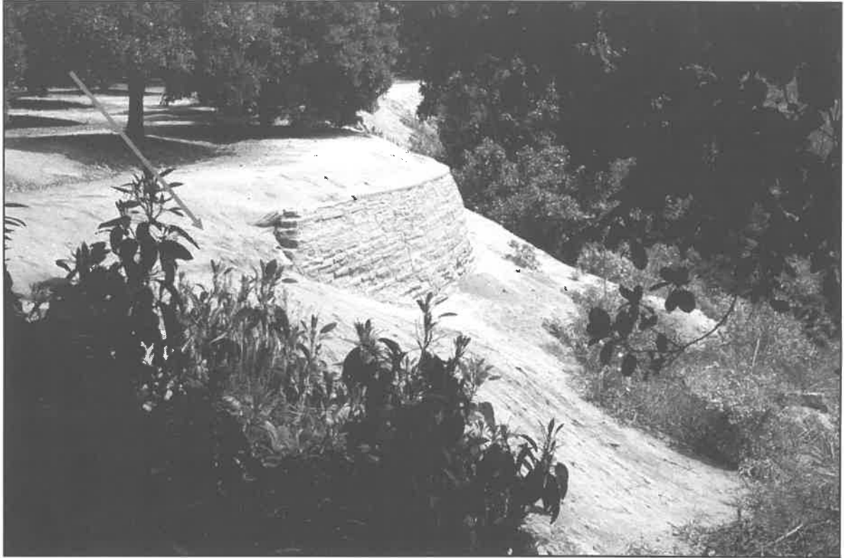
Image068.jpg: View of stacked cement block portion of site. The poured concrete section begins just left of the eroding gap indicated by the red arrow.
