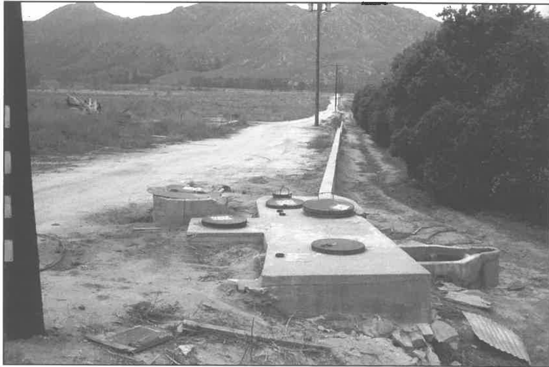
Image014.jpg: View of northern end of site to the south showing Feature 1: the RHCW conduit portal (larger manhole cover) and smaller orchard standpipe portals. The Feature 3 (retaining wall) extends to south. The buried RHCW conduit runs downhill beneath groves in the upper right.
